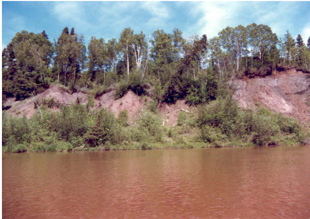
Figure 4. Slope failures along the Kaministiquia River in Thunder Bay, Ontario.
